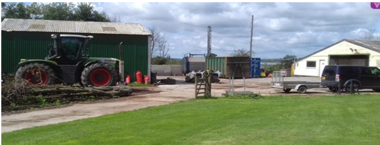
Photo taken on site of the boiler (and control room) and drying containers with two existing agricultural buildings either side – with 4m high flue (summer of 2022)
