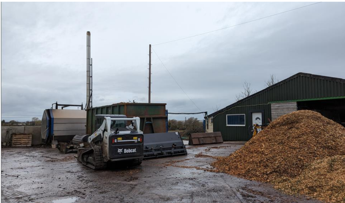
Photo taken on site of the boiler with the recently installed 6m high flue (and control room) and drying containers with the former piggery on the right
